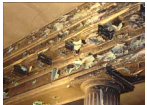
Fire damage to the interior.
