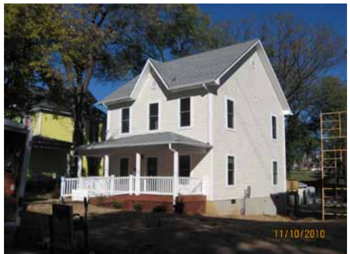
New construction at 1713 Rorer Avenue. All photographs courtesy of Habitat for Humanity of the Roanoke Valley
